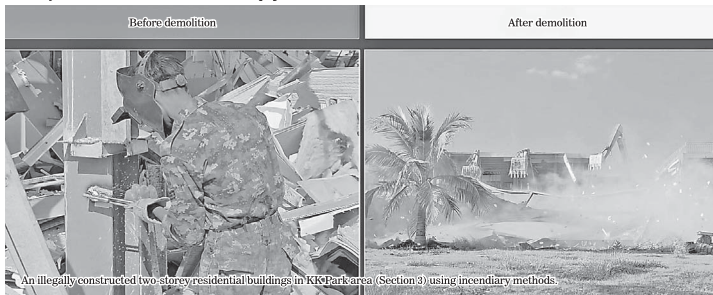
Demolition of illegally constructed two-storey residential buildings in KK Park area (Section 3)
