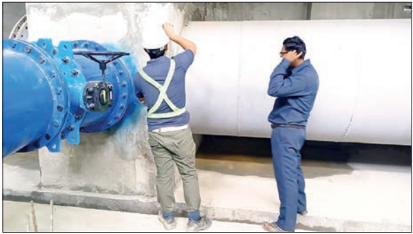
Officials inspect facilities inside the Hlawga Water Pumping Station.
