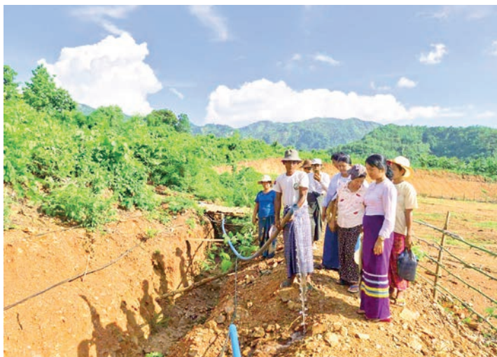
Officials inspect the ongoing water pipeline installation project in Yamethin Township, Mandalay Region.
