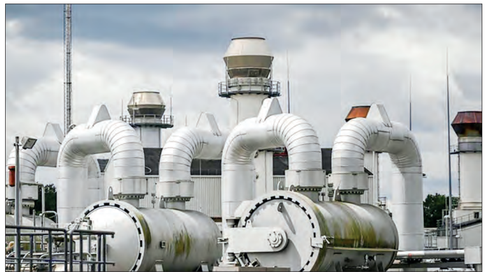
Pipes and pressure gauges for gas lines are pictured at Open Grid Europe (OGE), one of Europe's largest gas transmission system operators, in Werne, Germany on 15 July 2022. PHOTO: AFP/FILE
