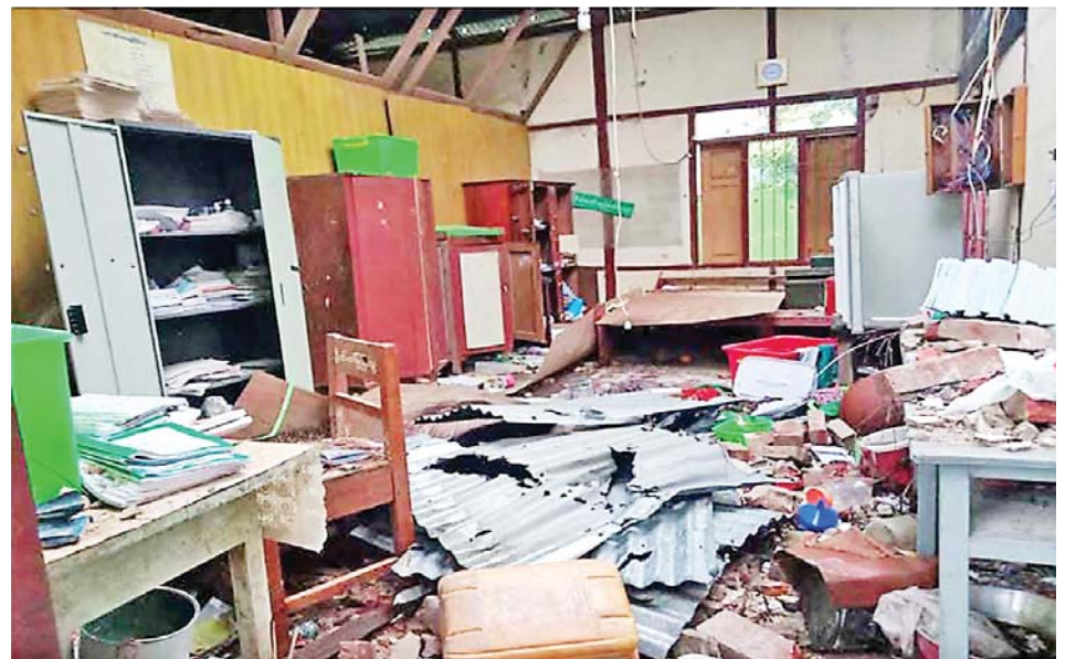
A school building, destroyed by terrorist insurgents.
