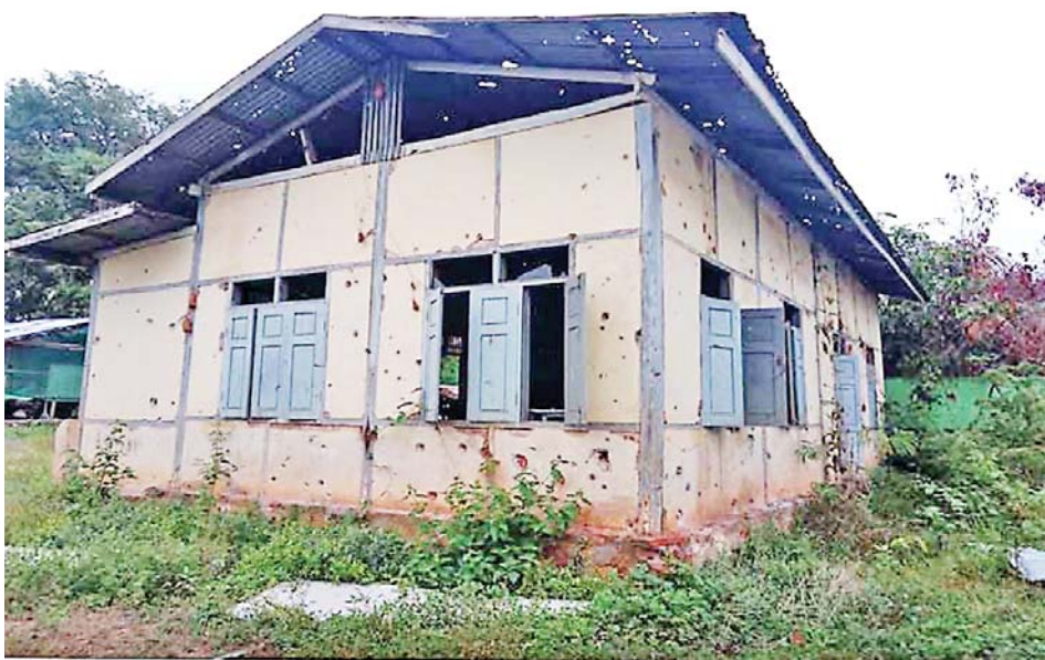
A school building, destroyed by terrorist insurgents.
