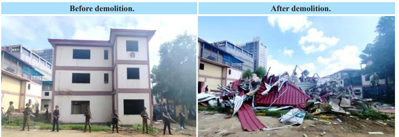
Demolition and destruction of illegal buildings used for operating online gambling with heavy machinery in Shwe Kokko area, Myawaddy District, Kayin State.
