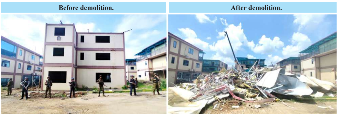
Demolition and destruction of illegal buildings used for operating online gambling with heavy machinery in Shwe Kokko area, Myawaddy District, Kayin State.
