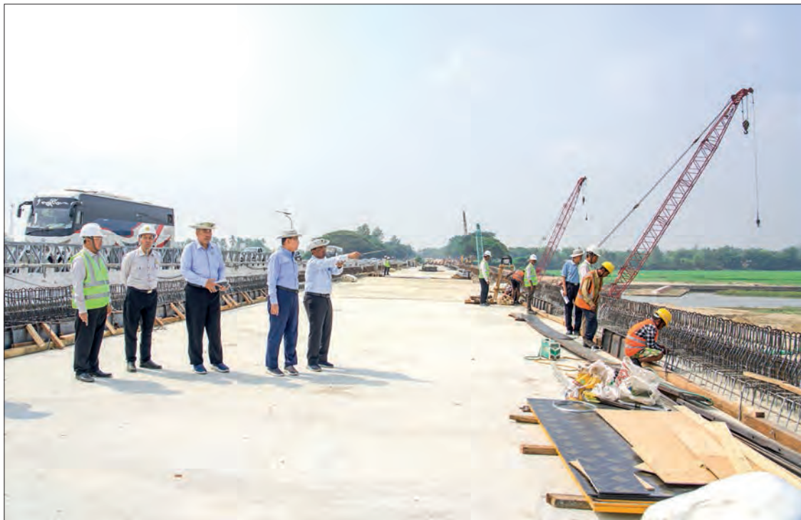
Union Minister for Construction U Myo Thant inspects the repair of the Swa Creek Bridge on the Yangon-Mandalay Expressway (Nay Pyi Taw-Yangon section).
