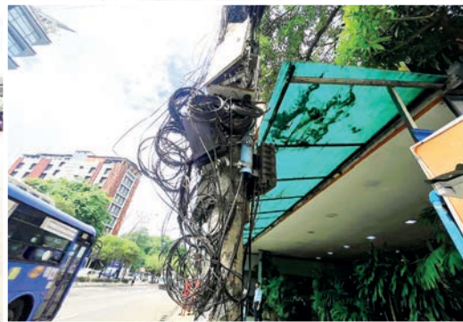
Images capture communication cables installed across Yangon Region.
