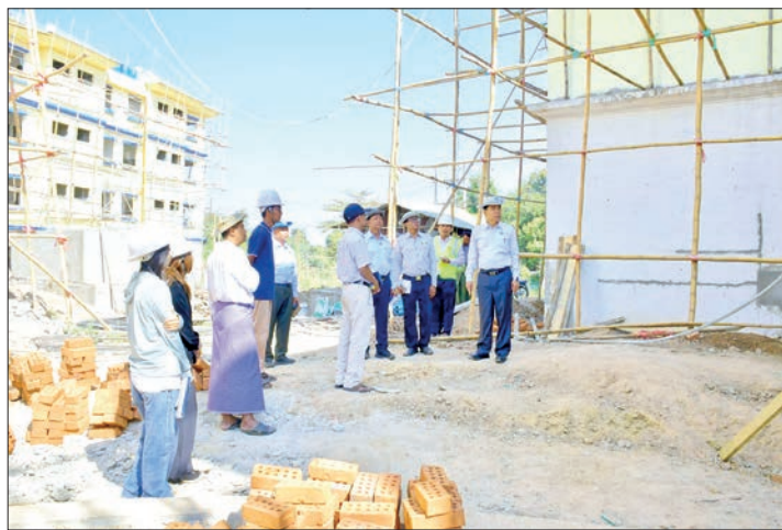
Officials inspect staff housing in Nay Pyi Taw, where major renovation works are underway.
