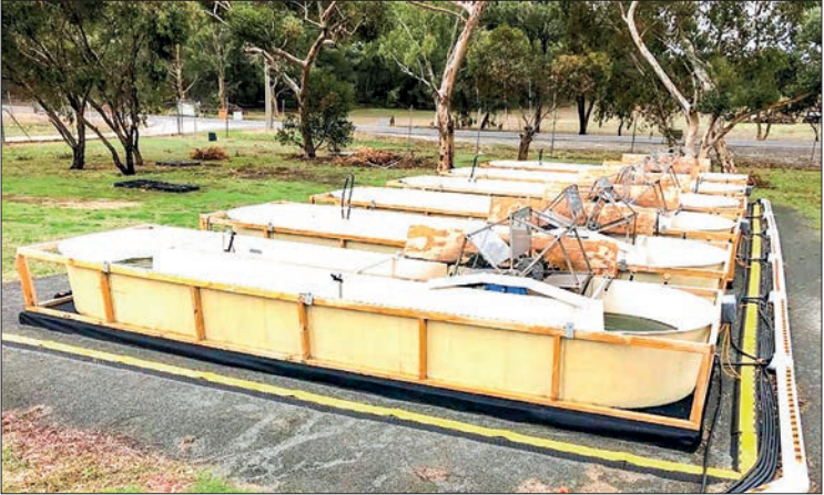
This photo taken on 11 June 2025 shows "sequencing batch reactors" treating effluent and removing biosolids at a wastewater treatment plant in the Barossa Valley, South Australia. PHOTO: FLINDERS UNIVERSITY/HANDOUT VIA XINHUA
