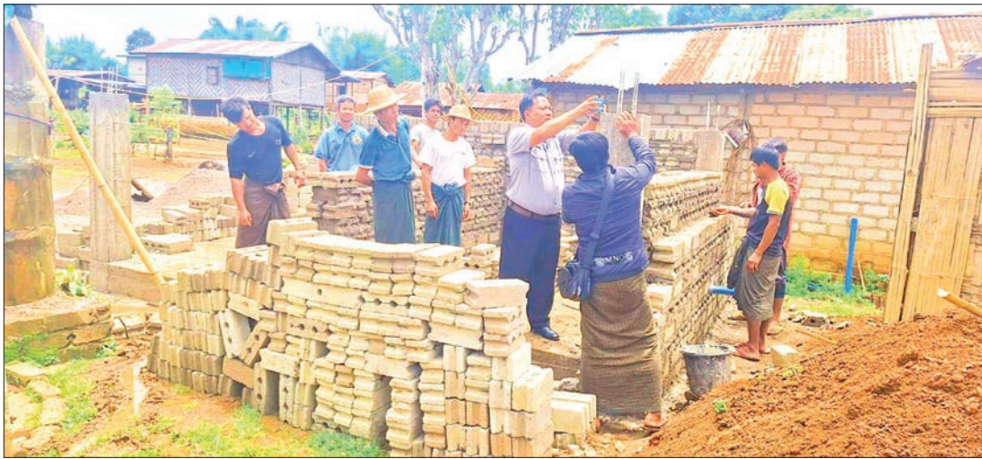
Officials inspect the progress of development work in Khaehpaha Village, Nawngkhio Township, Shan State (North), yesterday.
