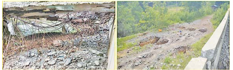
Destruction of Five-Pole Bridge along the Kyondo-Kawkareik-Thingannyinaung road by terrorist insurgents using landmines.
